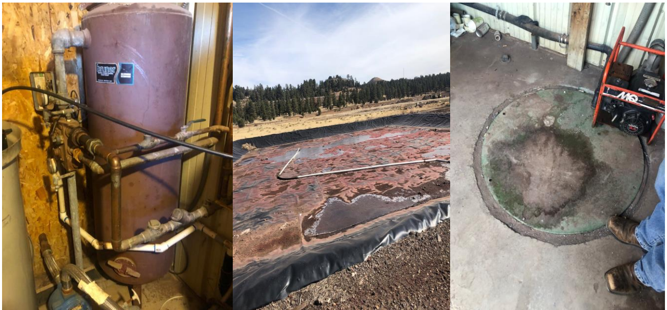
Figure 3-5: Grand Canyon Railway's current softener column, rainwater reservoir, and grinder pump location.
